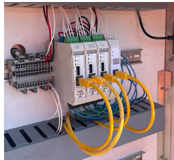
Image 1: Equipment at the site
