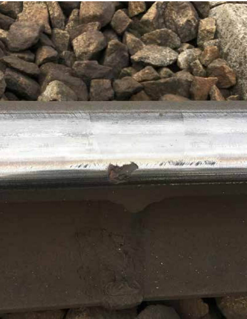
↑ Even minor defects like this rail head crack have already been detected using FTS.
